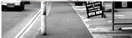
Patchy pavement surfaces
